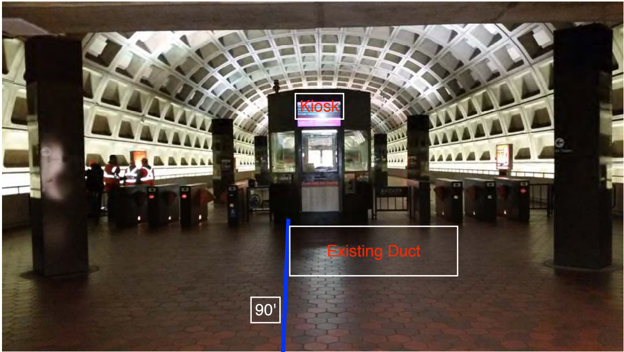
Photo #1: Existing duct layout on mezzanine floor
